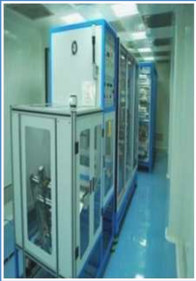
Pulse Capacitor Development Facility
